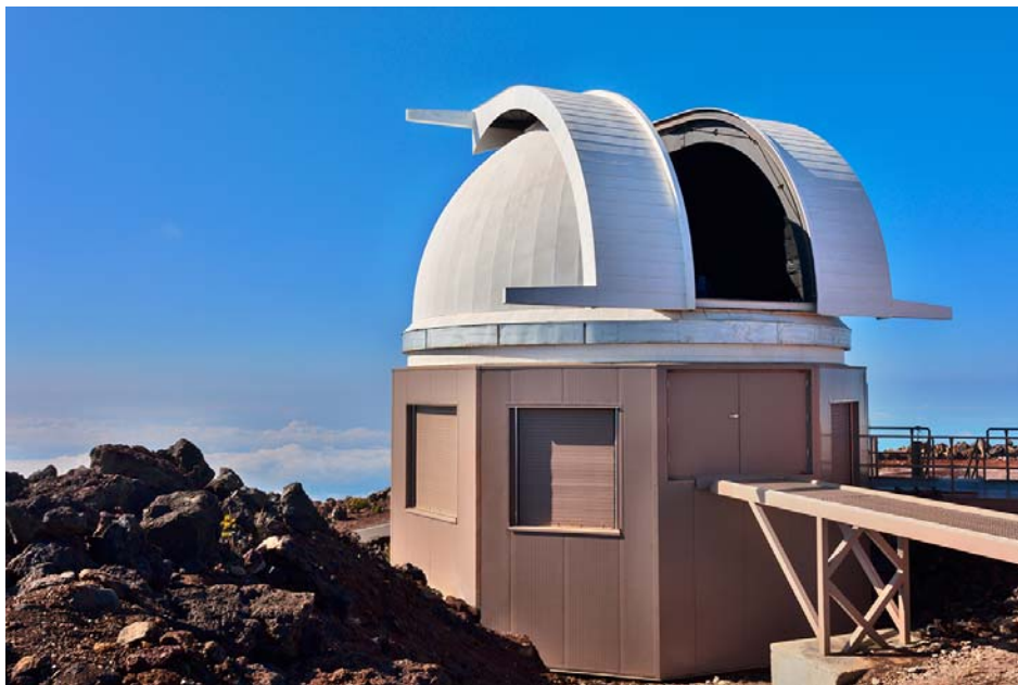
Figure 3. The new exterior panels and vent doors after the completion of Phase 3.
