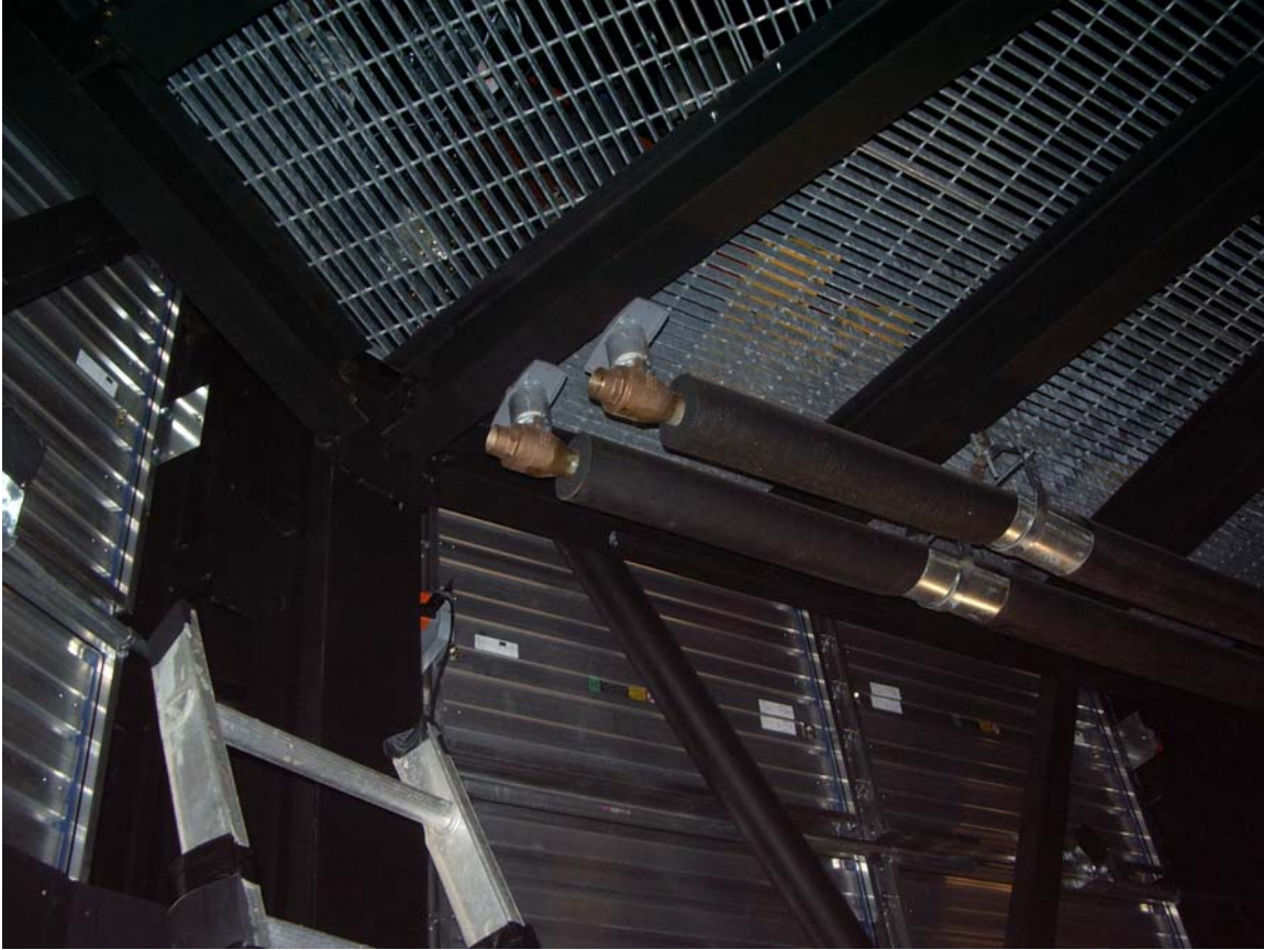
Figure 5. The existing termination of the FC-2 piping.
