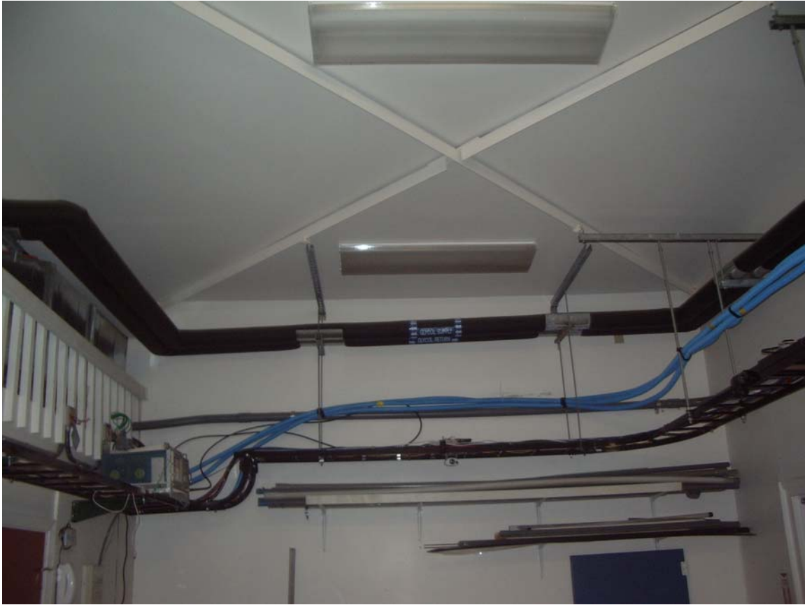
Figure 6. The support building chilled water lines that need to be replaced are shown near the top of this photo (see drawing MP101).
